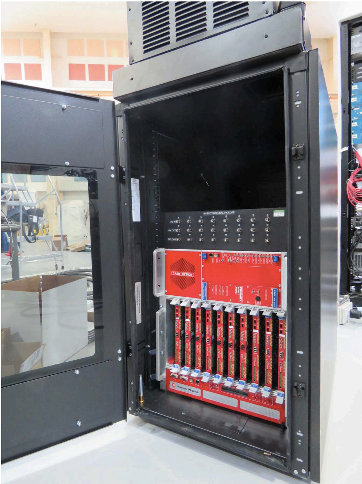
Figure 4: The CAEN electronics have been assembled in the cooling rack.
