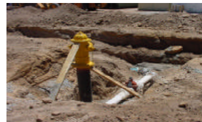
Hydrant, PIV and Thrust Block May 24, 2002
