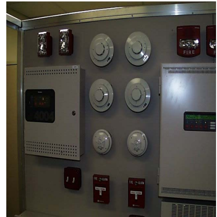
Facility Systems Laboratory at LANL
